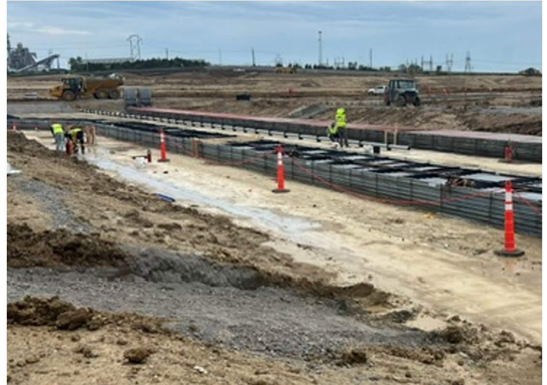
UG utility in RICE Engine Hall – below foundation
